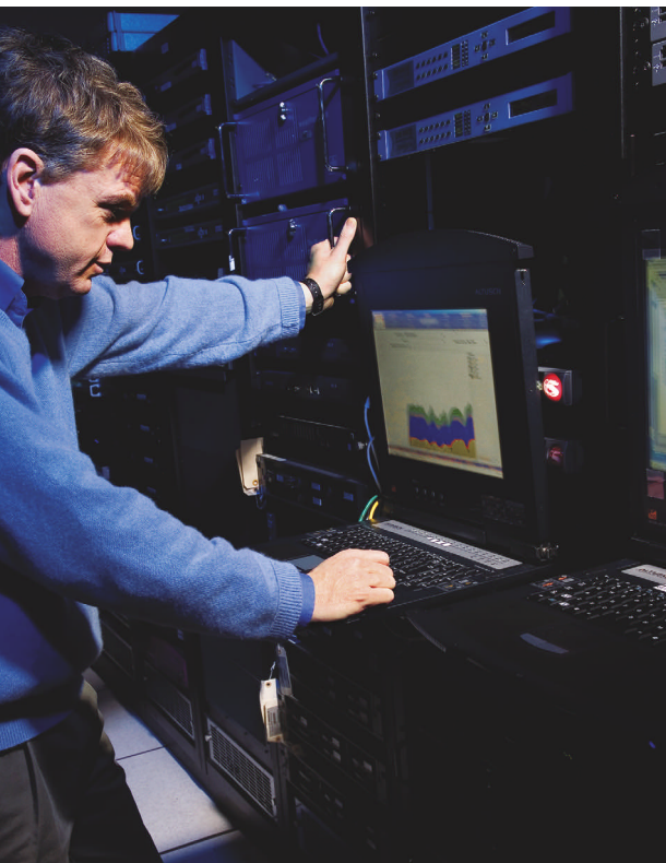
Bill Downey tests equipment at the ends of a video-distribution network.
